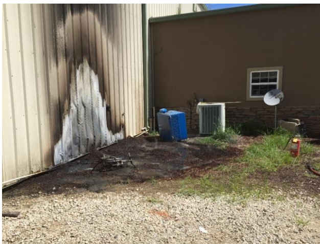
Fire due to an electrical short in external outlet burning a bicycle, mat, and other materials next to wall.
